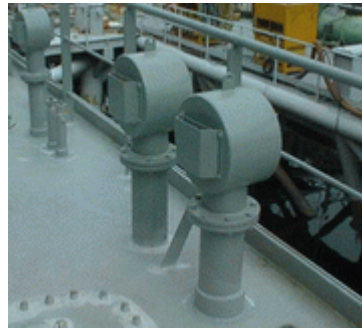
11. All air pipes and ventilators on the fore deck (forward 25% of ship's length), all air pipes to day tanks and selected air pipes and ventilator coamings aft of the forward 25% of the ship's length.
